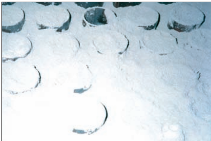
Air preheater, after four months process without Sonic Cleaning. The entire boiler has to be shut down at this time.
